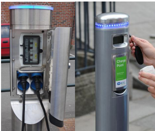
Figure 4: Left- 'dumb' charging point, Right – 'smart charging point
