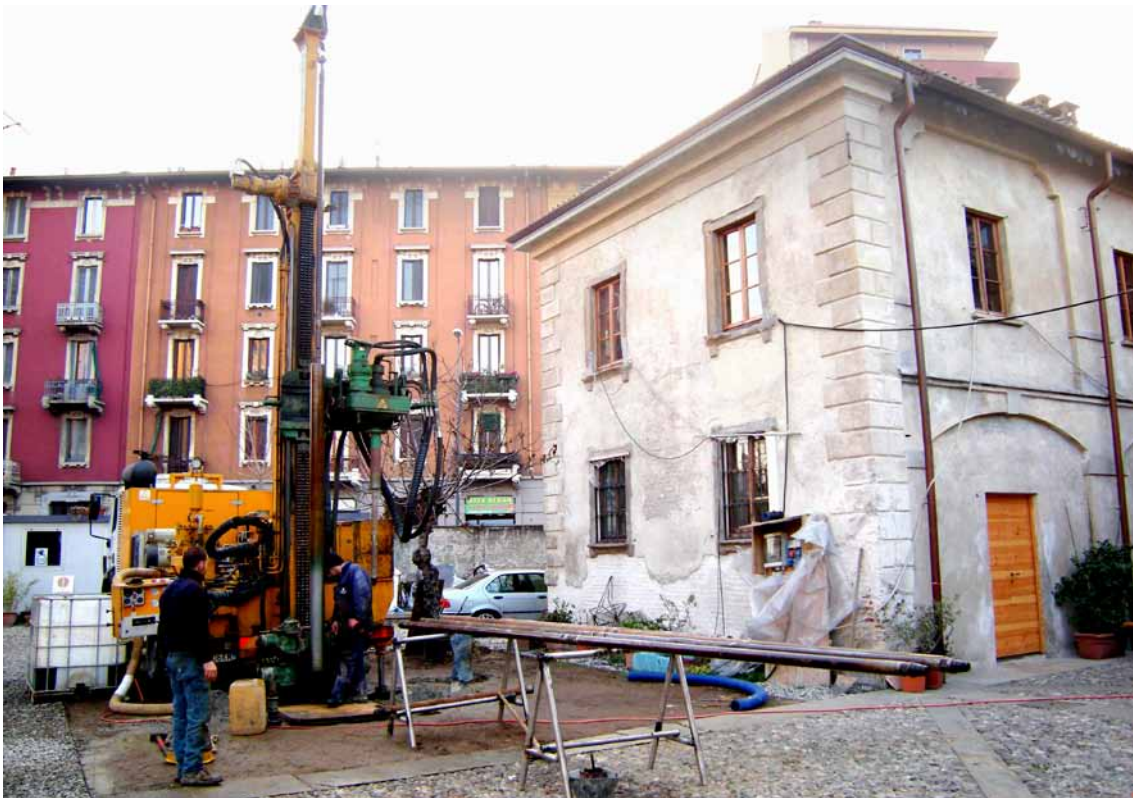
Cascina Cuccagna, Milan, digging the wells to connect the heatpumps to underground water table. Photo: Courtesy of Cascina Cuccagna
