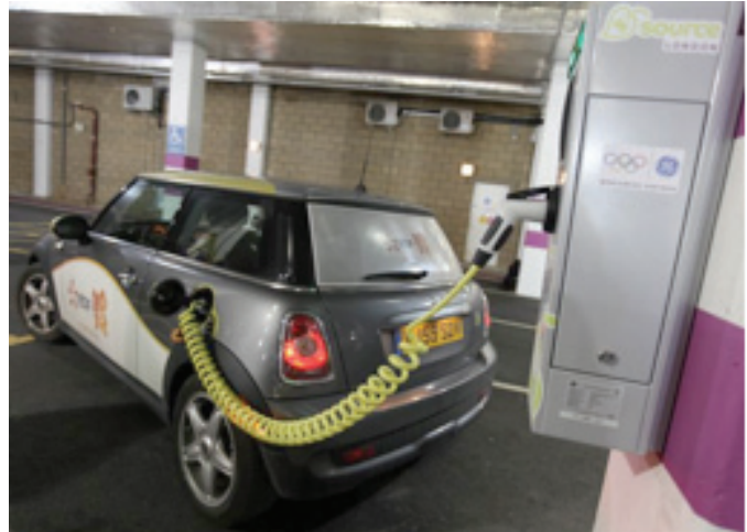
Charging of Electric Vehicle Photo: Transport for London (TfL)
