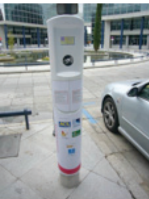
On street charging point - Madrid
