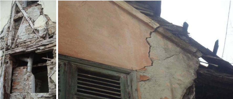
Fig. 16 Common damages of mud brick masonries in Veria
