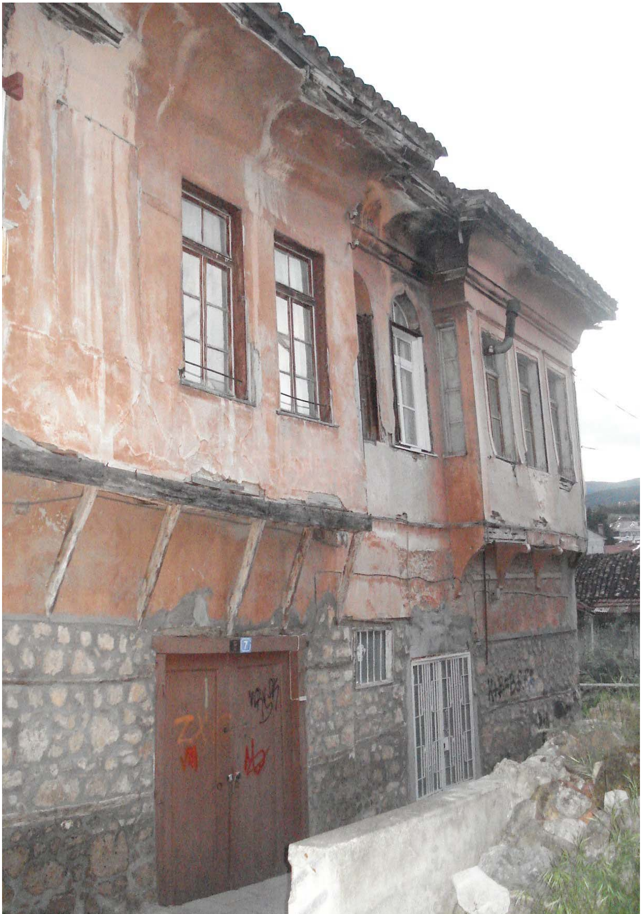
Figure 3: Beautiful old house in need of restoration
