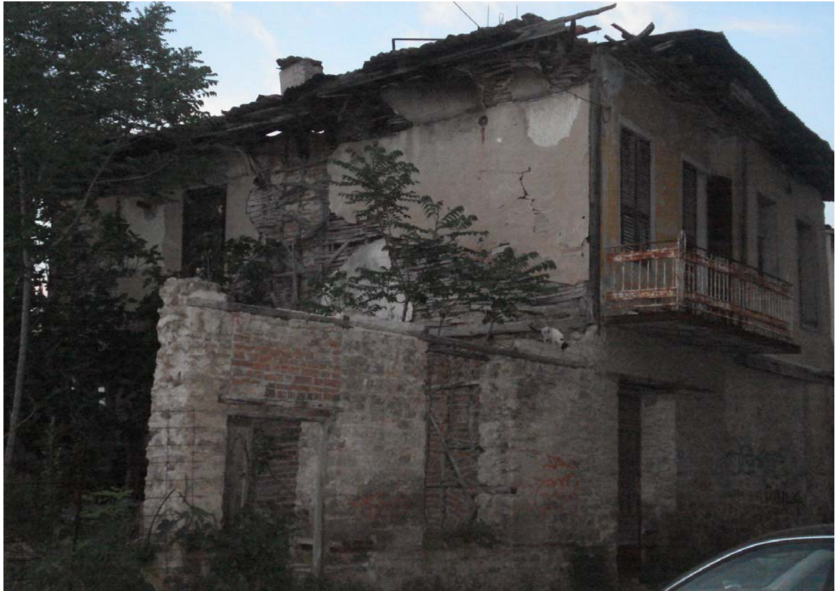
Figure 1: Dilapidated building in the city center of Veria
