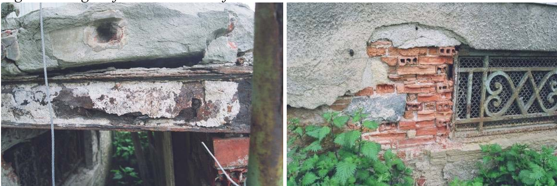
Fig. 8 Detachments in old building due to corrosion of metallic element
