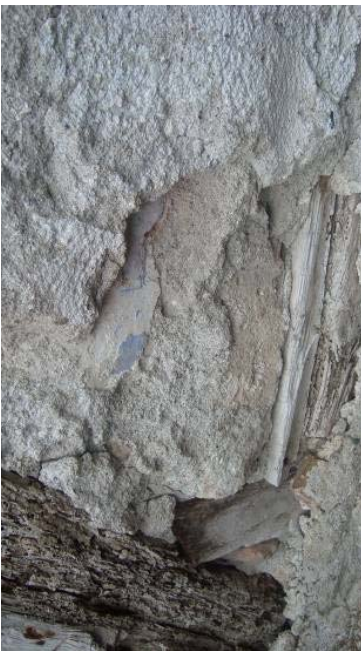
Fig. 17 Unsound wooden beam in old earth building
