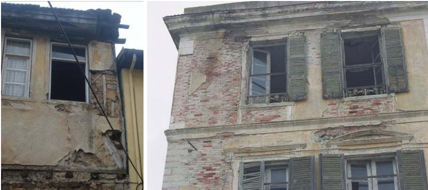
Fig. 2 Common damages of old structures in Veria
