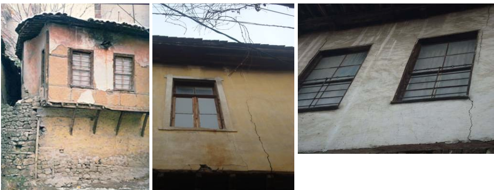
Fig. 15 Common damages of mud brick masonries in Veria
