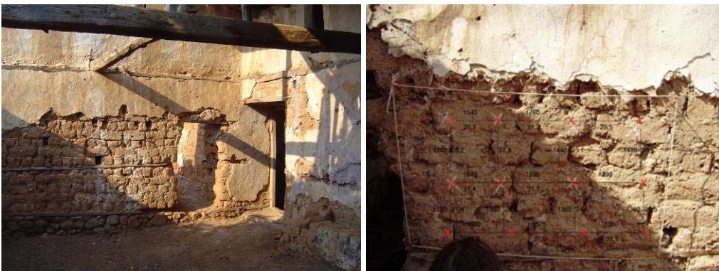
Fig. 21 Selection of a wall with cracks for the injection with soil-based grouts
