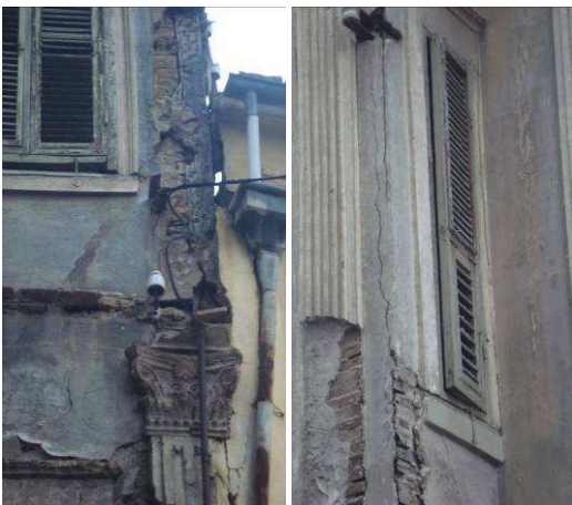
Fig. 7 Damages of external walls of an eclectic old house in Veria
