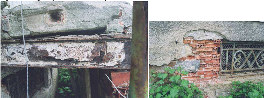
Fig. 8 Detachments in old building due to corrosion of metallic element
