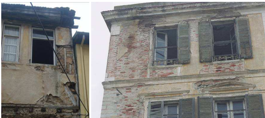
Fig. 2 Common damages of old structures in Veria
