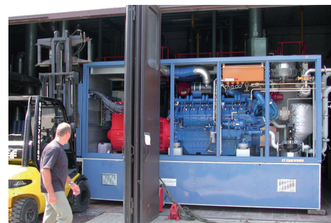
CHP motor 611 electrical kW, 800 thermal kW power gas engine for district heating network, Sossenheim, Frankfurt, Germany.
