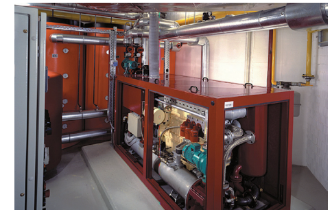
50 electrical kW motor managed by social home owners association Rödelheim, Frankfurt, Germany.
