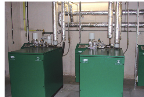
Cogen motor 5 electrical kW SENERTEC 'Dachs' machine, Frankfurt, Germany.
