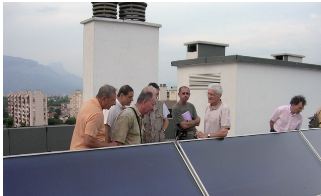
Solar water heating system, Echirolles, France.
